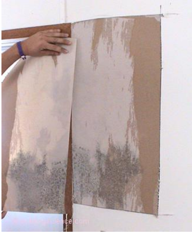
Photograph 6: Vinyl Covered Gypsum Board —FEMA trailers are lined with vinyl-covered gypsum board as are HUD manufactured houses. This leads to mold problems. The only solution is to not install vinyl covered gypsum board.
