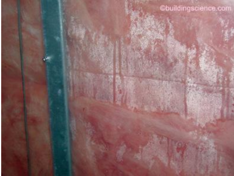
Photograph 9: Condensation on Polyethylene Vapor Barriers— Solar driven moisture out of reservoir claddings can lead to cavity side condensation on polyethylene vapor barriers in cold climates such as Chicago.
